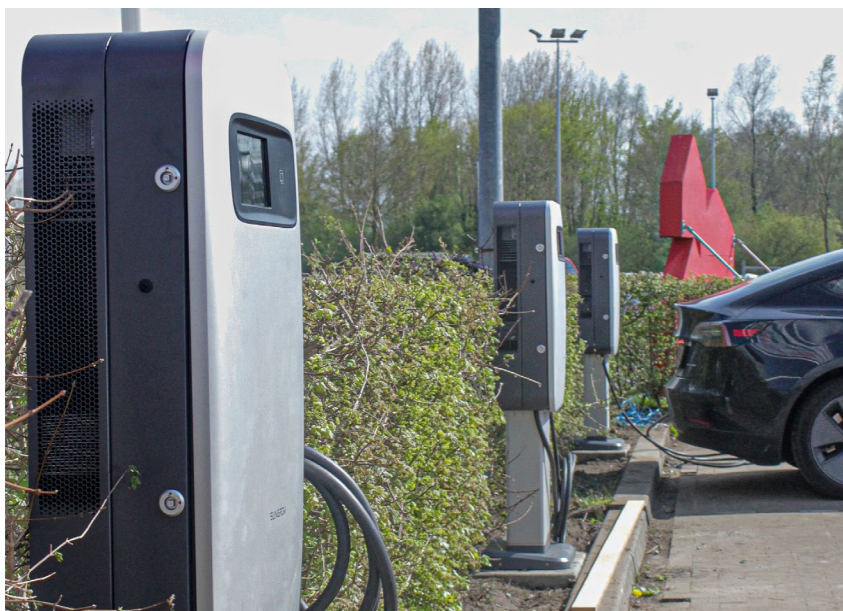
Fast Charging while shopping in Groningen, Netherlands: ten IDC30E pole-mounted DC Chargers
