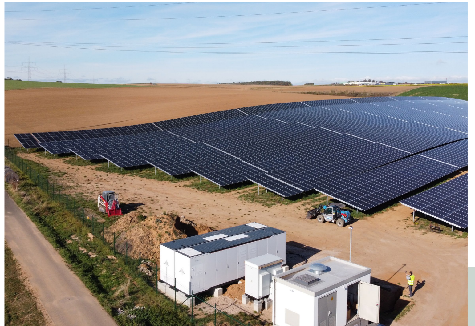
Solar plus Storage in Theilheim, Germany: A ground mounted system with one SG3125HV-30 inverter and two Sungrow PowerTitan ST2752UX storage systems
